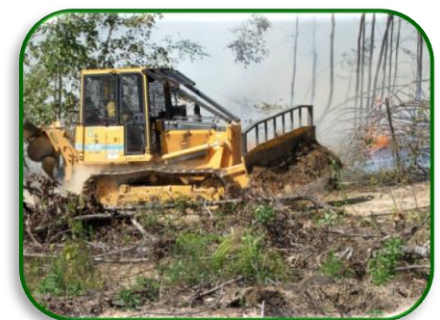
Figure 2: MFC Fire Unit. Photo by Bill Kitchings.
